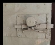
"Doors to Manual"
